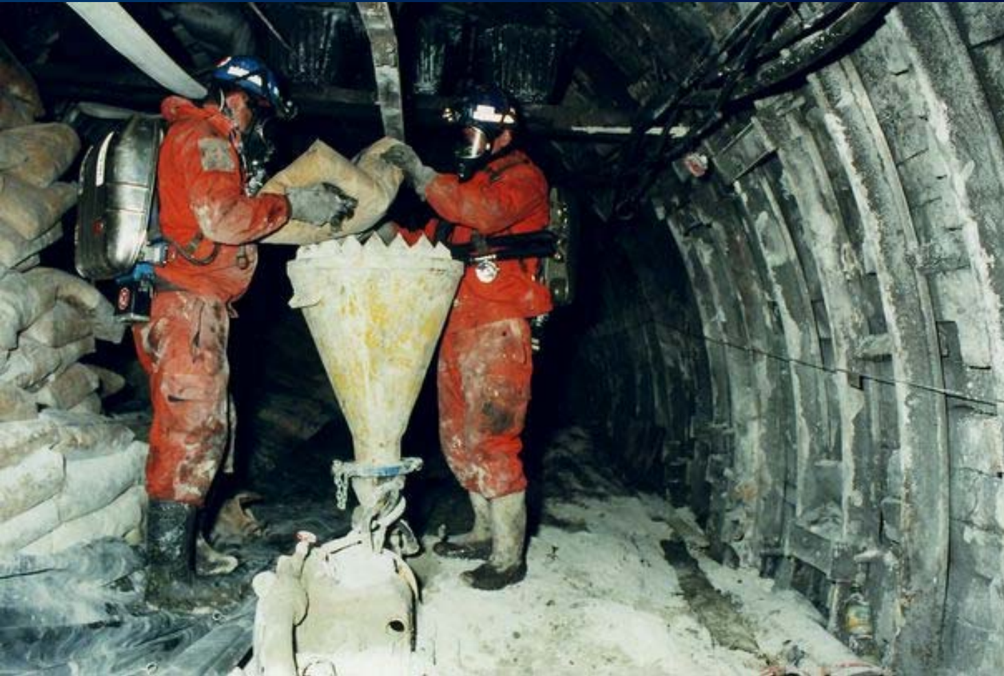
BUILDING OF A PLASTER DAM DURING A MINE FIRE WITH SCBA BG174
